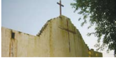
This church near Sharakpur was damaged in a confrontation between Christians and Muslims in August. Through the Fellowship of Christ we will provide funds to repair the church.
